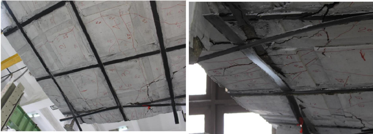
Fig. (9): Pattern of Crack, Debonding of FRP for BS1.
