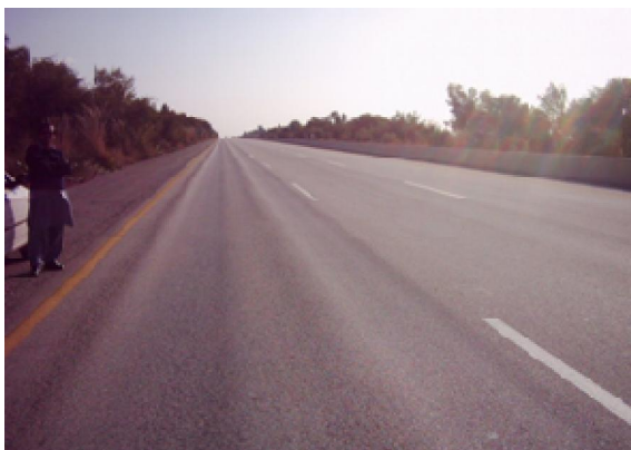
Figure 1. Severe Rutting on Motorway M-1
