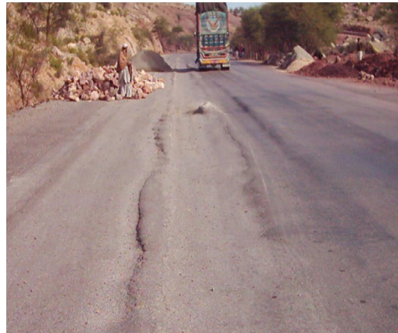
Figure 2: Rutting in Asphalt Layers due to Heavy Loading
