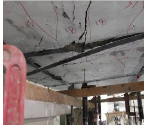
(a) Concrete Crushing and Debonding of FRP for Bonded Slab with CFRP Strips (BSS).
