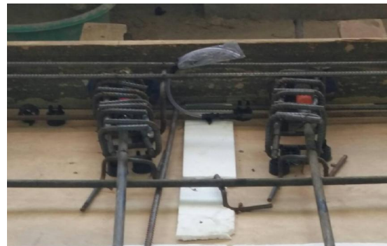
Fig. (6): Bursting Reinforcement
